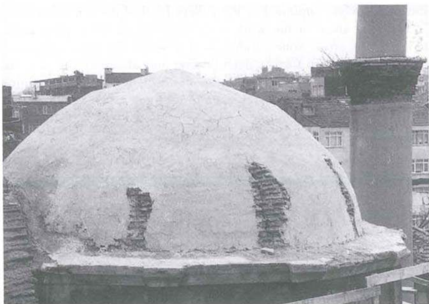
Figure 8. Zeyrek Camii, south church, cupola over the inner narthex with radial cracks at its base (A. Neftçi, 1998).
